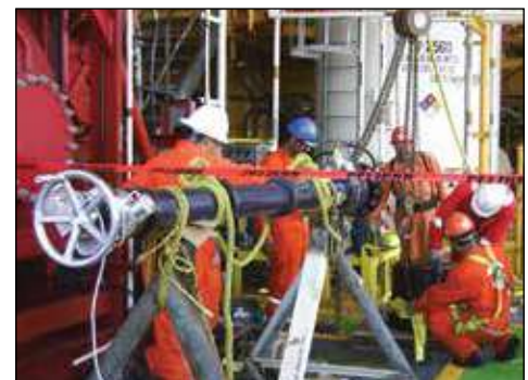
▼ CHT2000 hot tapping offshore application.
