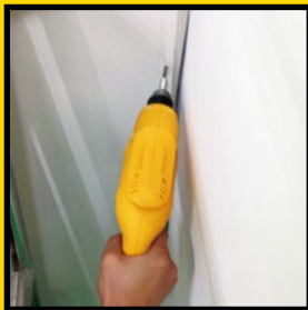
2 Driving Screws On Window Frame & Drill Holes In Wood Frame 10mm Rotary Drill STD5510
